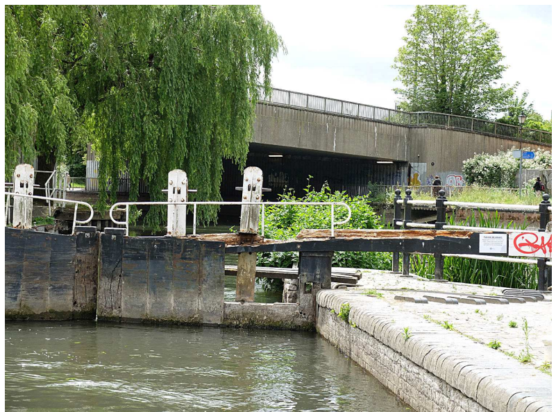
Above:- County lock in Reading only has a rise of 1ft the gate had a CRT apology notice to boaters on the rotten beam stating to be repaired soon.
