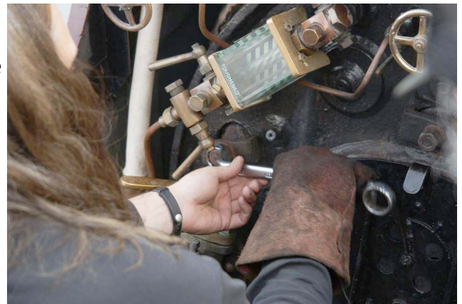
Releasing the mud doors on the boiler backhead
