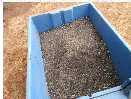
After all tubes were cleaned, this bucket shows how much soot/ash was removed from the smokebox
