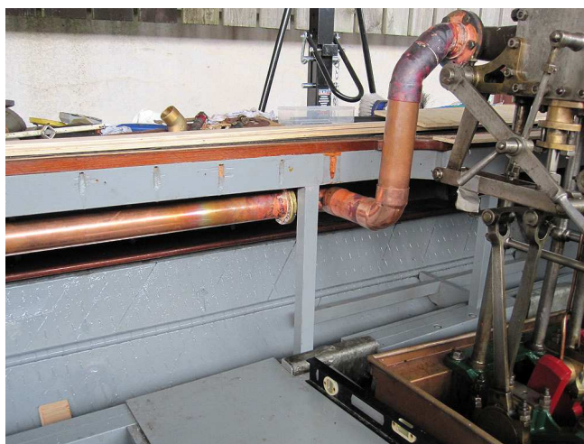
Photo shows route of new exhaust pipe
