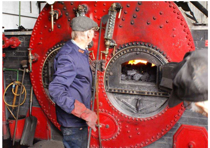
The Lancashire coal fired boiler in steam at Crofton. The coal used is ordinary household variety not steam coal
