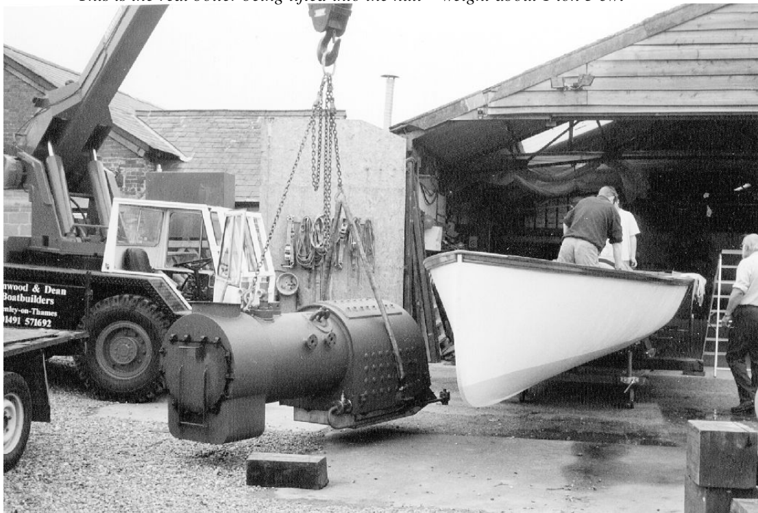
This is the real boiler being lifted into the hull – weight about 1 ton 3 cwt
