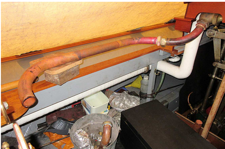
The long part of the engine steam pipe
