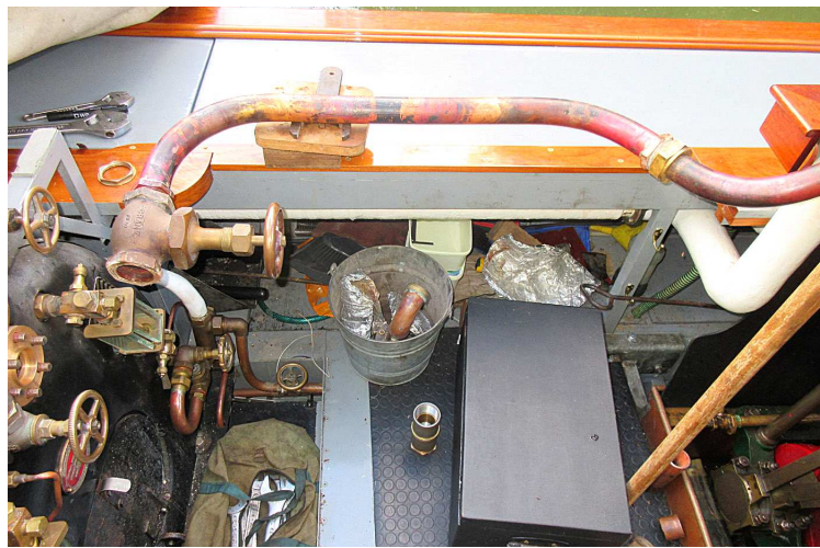
The main stop valve now fitted
